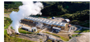
Te Ahi O Maui (TAOM) geothermal power plant (New Zealand)
