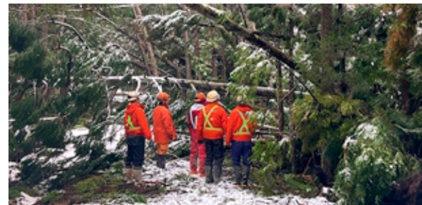
Preliminary survey of road opening work near the Mitsui Interchange on the Noto Satoyama Kaido
