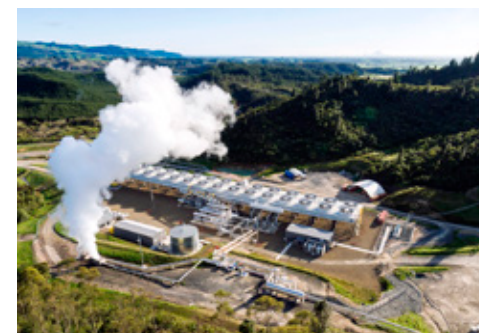
The Te Ahi O Maui (TAOM) geothermal power plant owned by Eastland Generation Limited (New Zealand)
