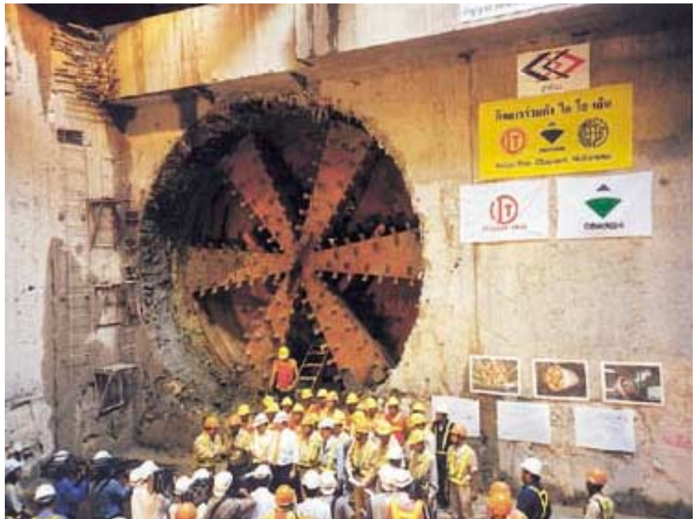
Metropolitan Rapid Transit Authority [MRTA], Initial System Project, Underground Structures — North (Thailand)
