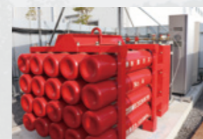
Hydrogen power generator
