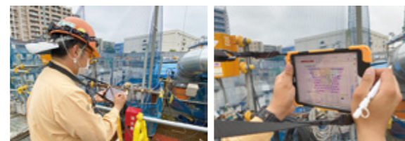
Real-time sharing of information with other employees and with suppliers and subcontractors by entering progress updates and corrective instruction into eYACHO® at construction site
