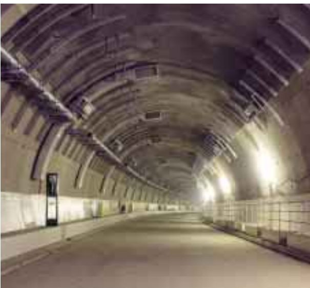
The Metropolitan Expressway Central Circular Shinjuku Route Naka-ochiai Shield Tunnel (outbound) Location: Tokyo
