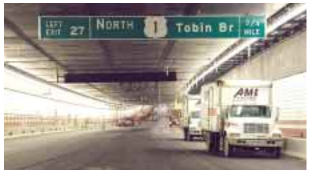
Central Artery / Tunnel project - I - 93 Tunnel Finishes (C17AA) in the City of Boston Location: Massachusetts, U.S.A.
