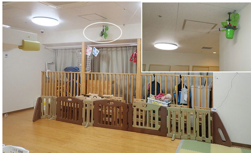
Installed plumbing connection style Multi Mist
