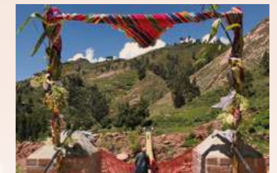
Project members built a bridge with steel beams and a wooden deck at a Bolivian mountain site more than 3,000 meters in elevation.
