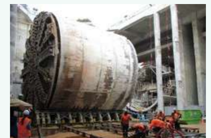
After drill-through was finished on the first tunnel, the shield machine was turned around inside the shaft and began drill-through on the second tunnel, shortening the construction period.
