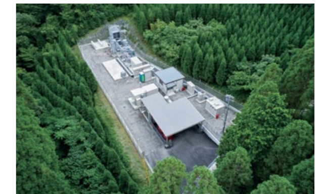
Geothermal power generation and hydrogen production plant on approximately 1,500m 2 of land in a mountainous area (photo: Quad, Inc.)
