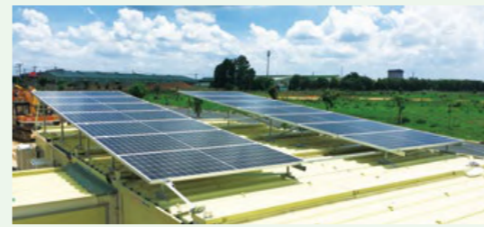
Solar panels installed on the roof of a construction site office
