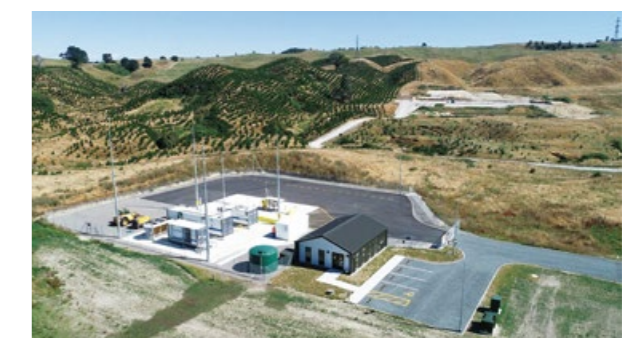
Hydrogen production plant located on the northern side of Lake Taupo where geothermal power generation plants are concentrated
