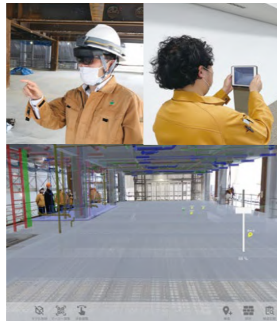
Conducting finishing inspection utilizing devices in the shape of glasses and in tablet form
