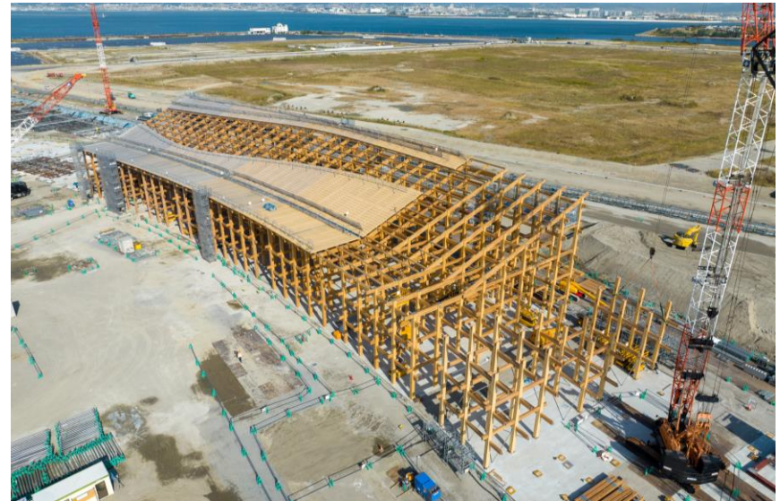
Construction status of the Grand Roof (Ring) at Pavilion World northeast section
